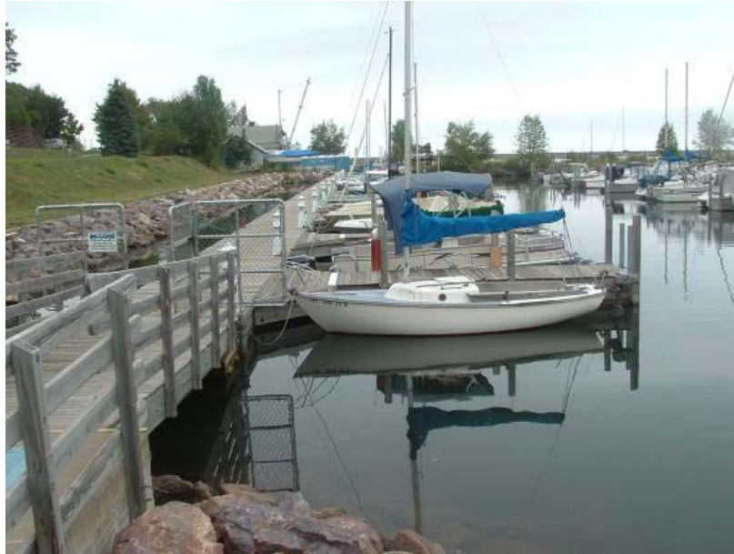
Figure 20. Floating docks can help marinas adapt to changing water levels. (Gene Clark)
