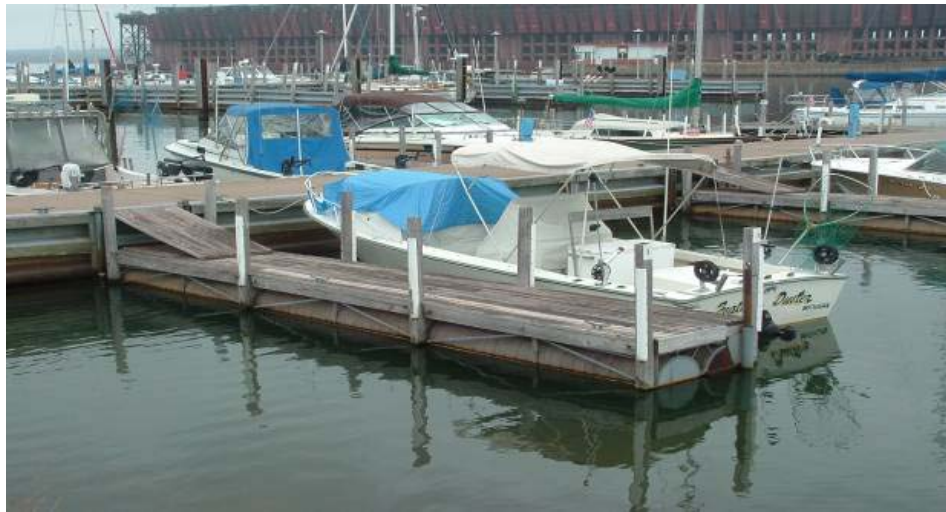
Figure 17. Low water can create safety issues when the distance from a fixed dock to the water increases. (Gene Clark, Wisconsin Sea Grant)
