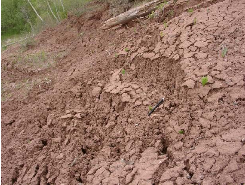
Figure 6. Severely fractured clayey till along the Lake Superior shoreline in western Bayfield County. These fractures fill with water in rainstorms, lubricating slide surfaces and creating instability on most slopes. (Source: D. Mickelson)
