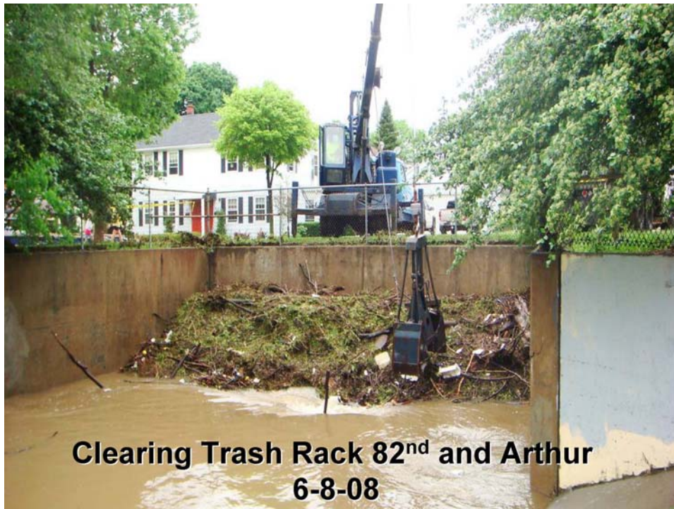
Figure 3. Debris from stormwater and flooding in Honey Creek inlet following torrential rains in June 2008. (Photo provided by the Milwaukee Metropolitan Sewerage District)
