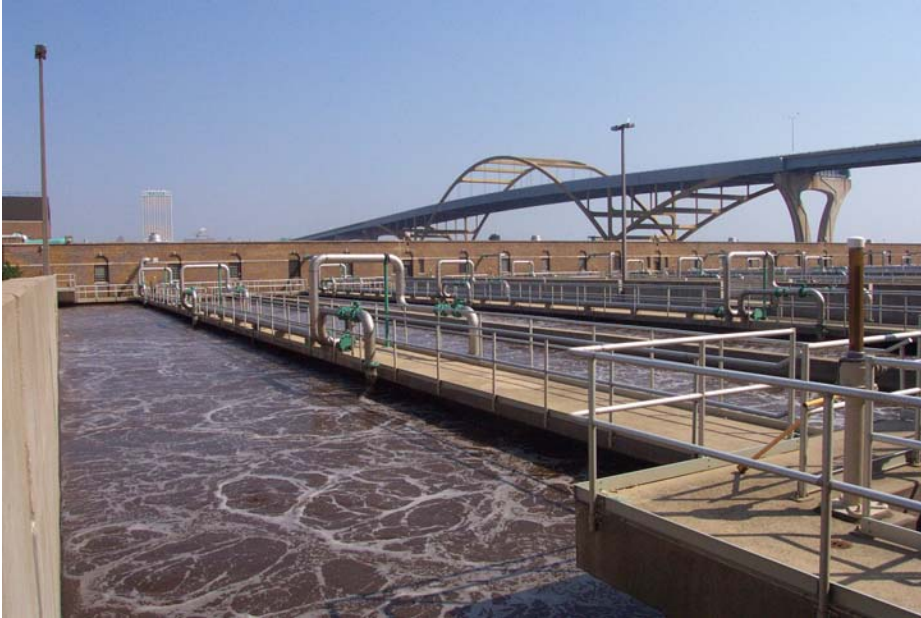
Figure 4. Jones Island wastewater treatment plant biological treatment aeration beds. High volumes at the plant following storm events may cause these reactors to washout, which would diminish treatment capabilities. Facility designs may need to consider additional capacity if climate changes alters storm patterns.
